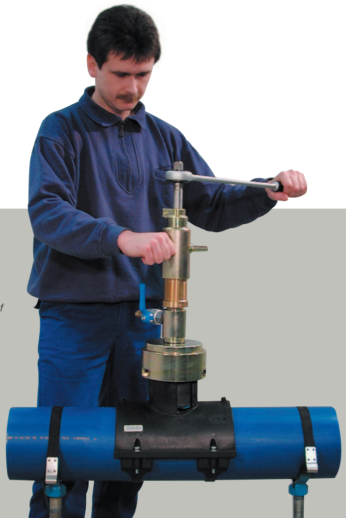
Picture 2: Direct, pressure free drilling of SA as reduced T-piece using drilling equipment by Hütz + Baumgarten
