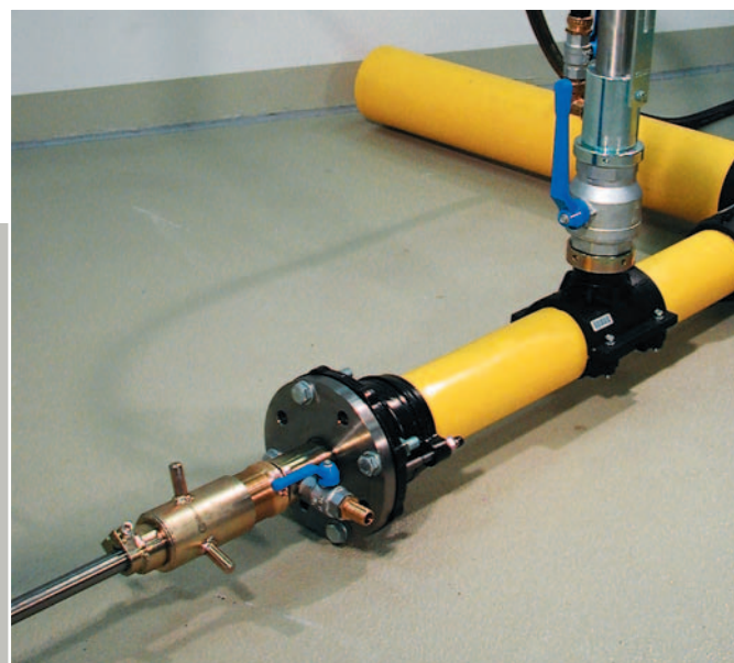
Picture 5: Drilling via AQUAFAST® clamp flange and FRIALEN® SPA shut off saddles with setting device
